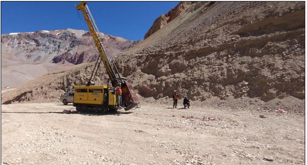
Figure 3: Drill rig setting up to drill the second hole at Tambo South (TMT-TSU-DDH002).
